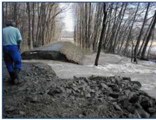
Fig. 3 Collapse of the Horka levee at the Morava River
