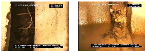
Fig. 4 The camera log of the pipe before the collapse
